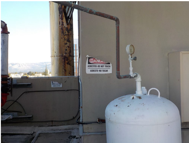
9. Wall Area on Roof Labeled as Asbestos
