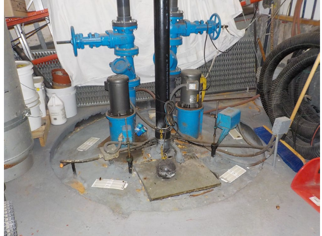
20. Sewer Sump in Basement
