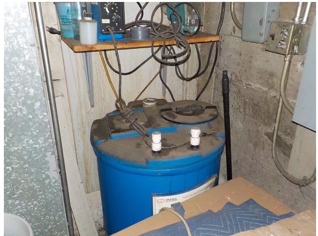
10. Cooling Tower Water Treatment Chemical Container in Rooftop Elevator Room Penthouse
