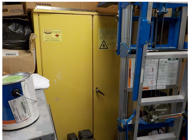
18. Flammables Cabinet in Basement Paint Room
