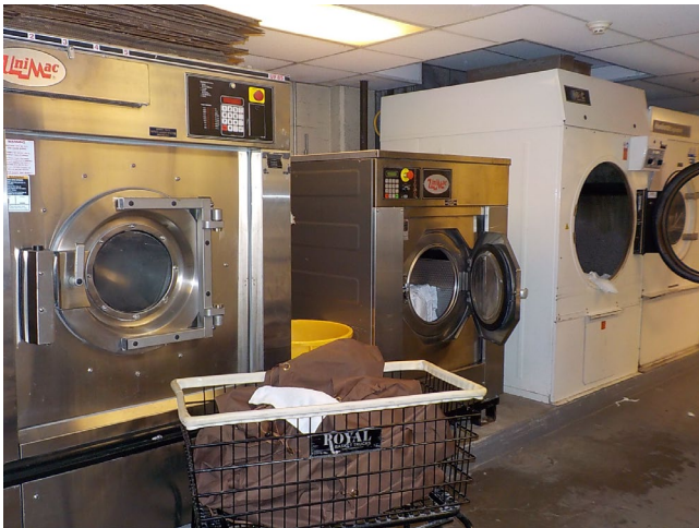
21. Basement Hotel Laundry Room
