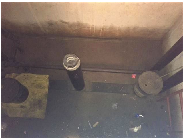
23. Hydraulic Kitchen Elevator Pit with Evidence of Previous Hydraulic Fluid Accumulation
