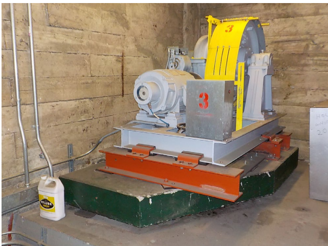
11. Traction Elevator Motor in Rooftop Elevator Room Penthouse
