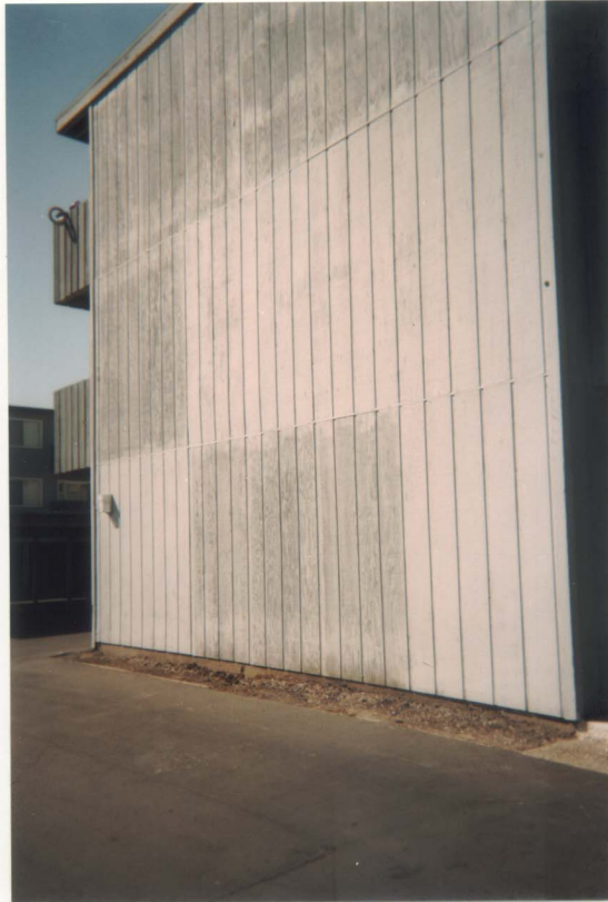
PHOTO 4: Patched T1-11 siding with old sheets exhibiting sun and moisture damage at south facades
