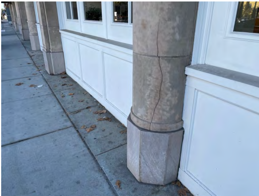
E - 28: Crack at column
