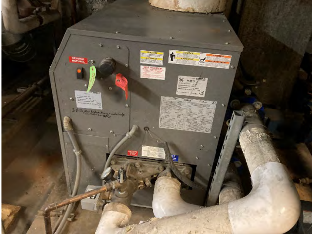
M-7. Space heating hot water boiler.
