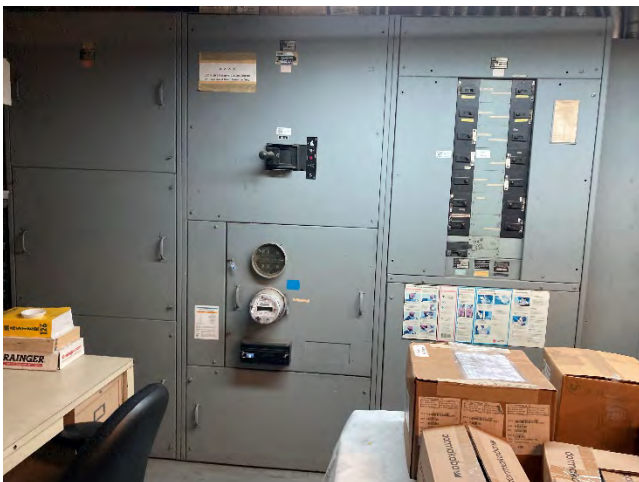
M-11. Main electrical switchgear.
