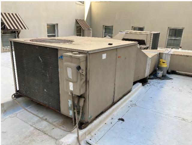
M-3. 10-ton packaged air conditioner.
