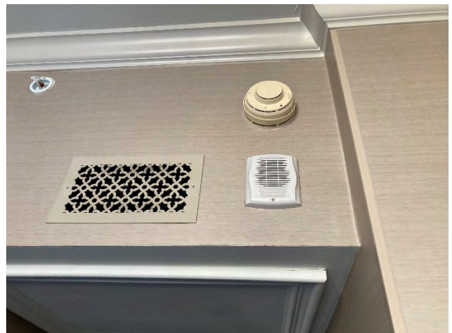
M-24. Guestroom smoke detector and alarm horn.
