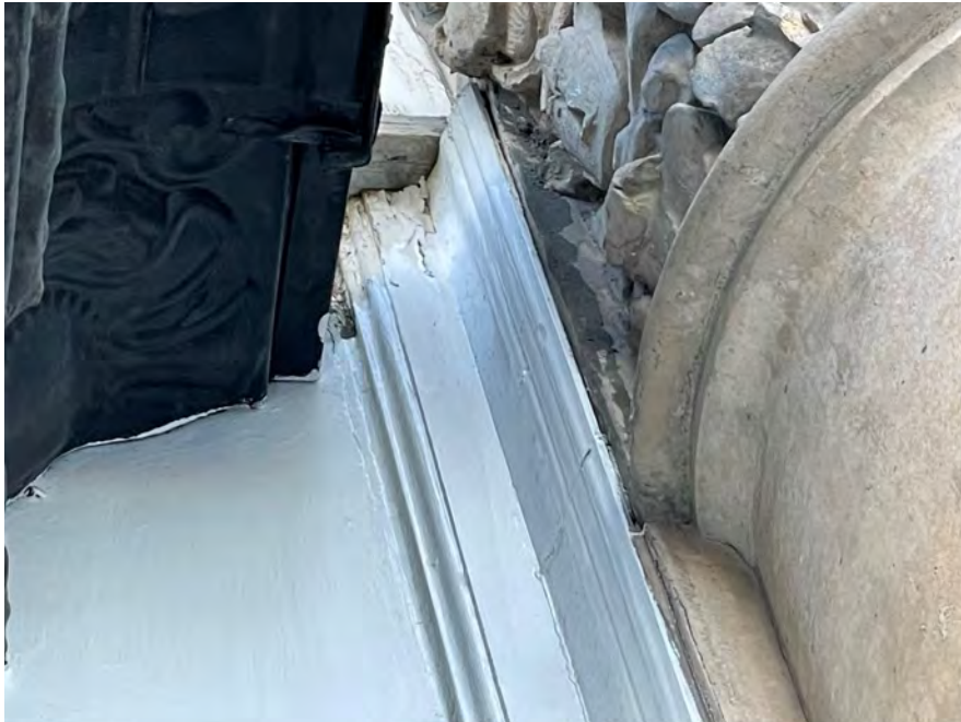
E - 30: Wood decay
