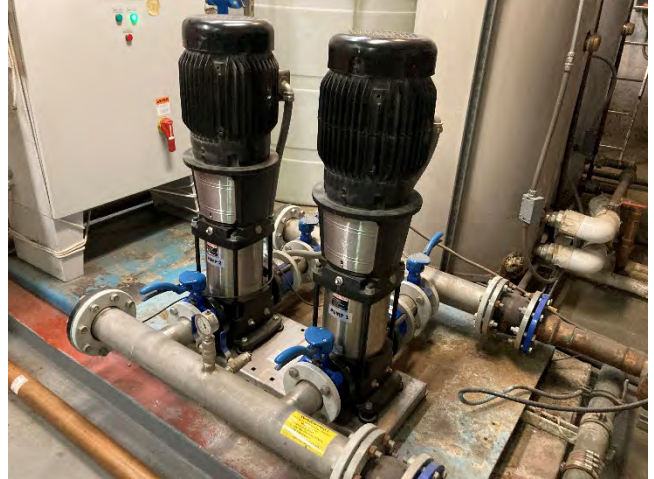
M-14. Duplex water pressure booster pumping system.
