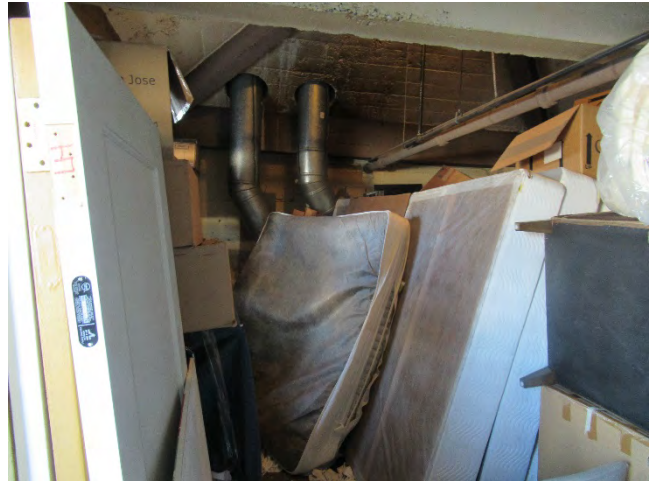
98. Inside the Penthouse on the northwest corner of the roof. The space is used for storage.
