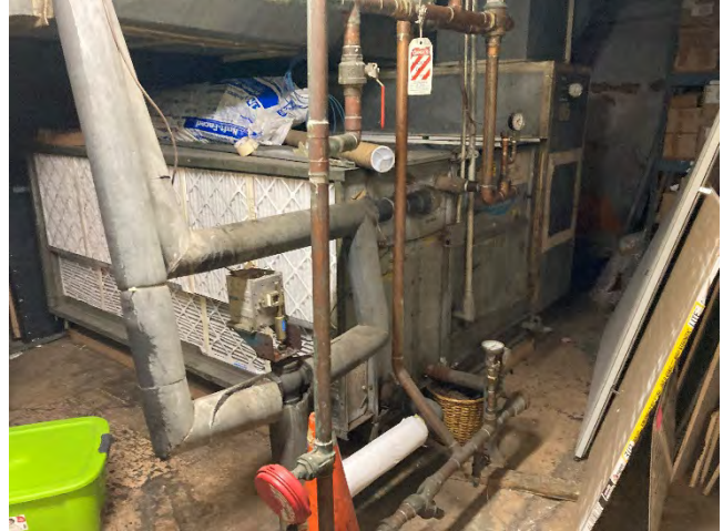
M-2. Lobby four-pipe fan coil unit.
