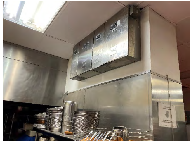
M-22. Kitchen hood fire suppression tanks.
