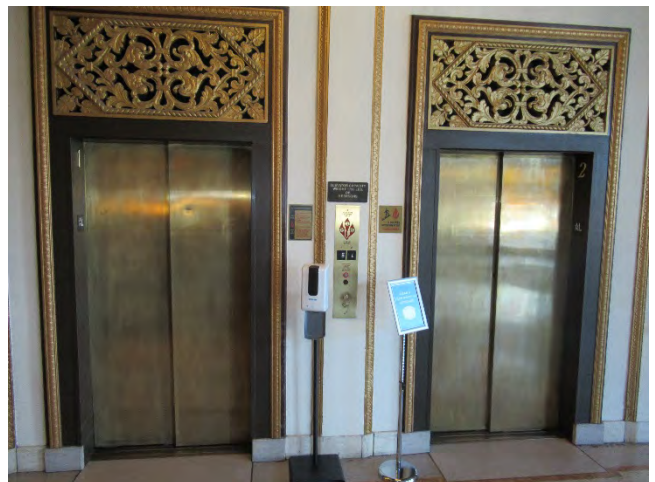
24. The two passenger elevators just east of the lobby. These elevators and the service elevator should have five-year load tests within the term of this report.
