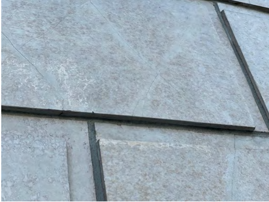
E - 29: Previously remediated cracks
