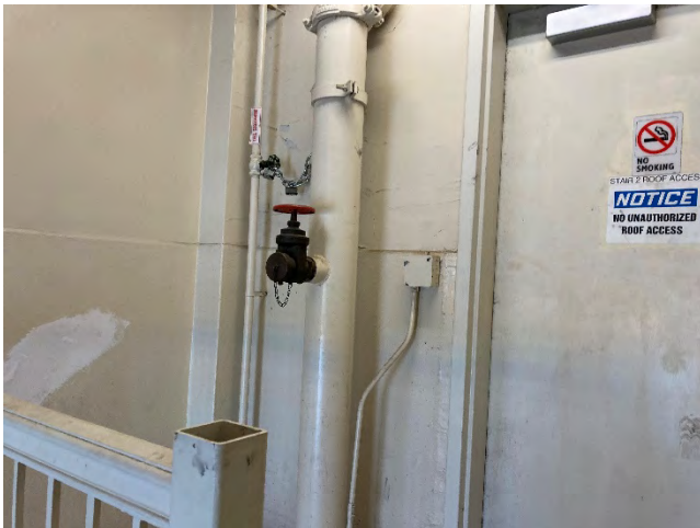
M-21. Stairwell standpipe with fire department connection.
