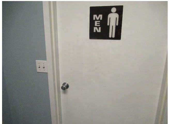
82. The door to the employee Men's Lockers and restroom. The door knob is Non-Accessible, and should be replaced. There is no Accessible jamb signage which should be provided.
