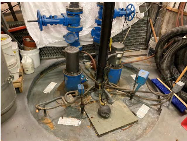
M-17. Underground parking garage duplex sump pumps.
