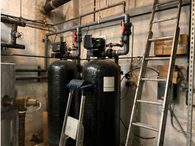
M-13. Water softener tanks.
