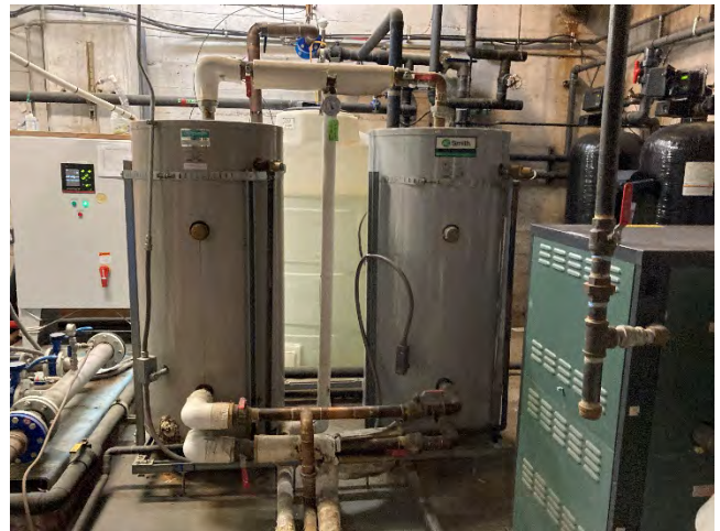
M-16. Domestic hot water insulated storage tanks.
