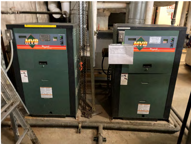
M-15. Domestic water boilers.
