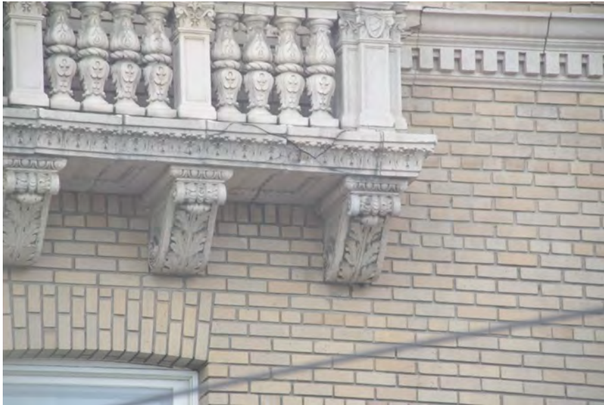
E - 31: Cracks at balcony
