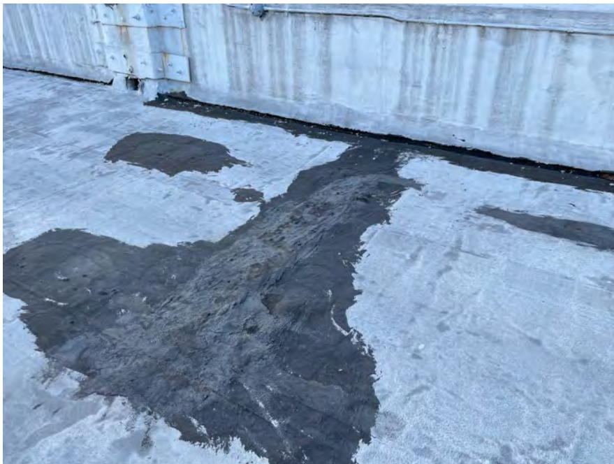
E - 2: Patch at Main Roof
