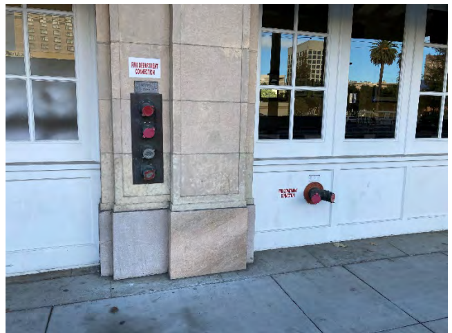
M-18. Exterior fire sprinkler and standpipe fire department connections.
