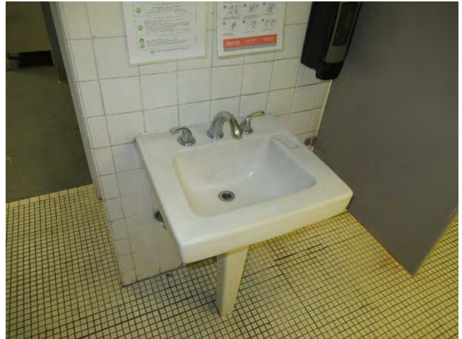
86. Lavatory in the men's locker bathroom. It should be replaced with one compliant for Accessible knee space.
