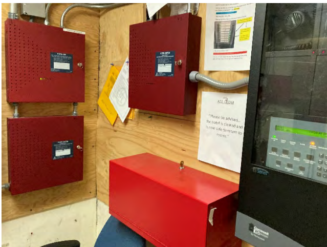
M-23. Building fire alarm panels.
