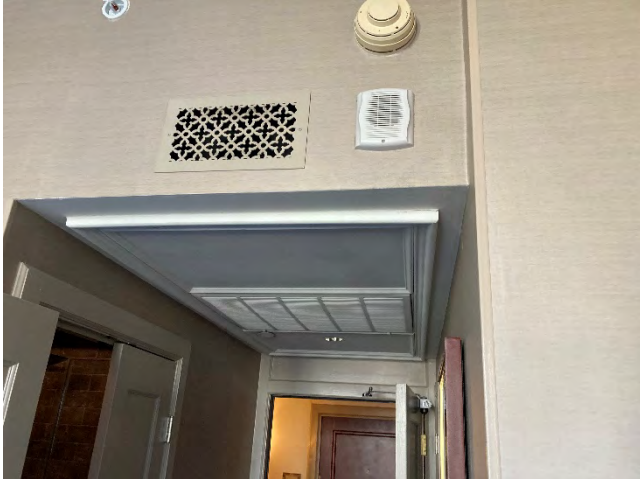
M-1. Guestroom water source heat pump supply grille.
