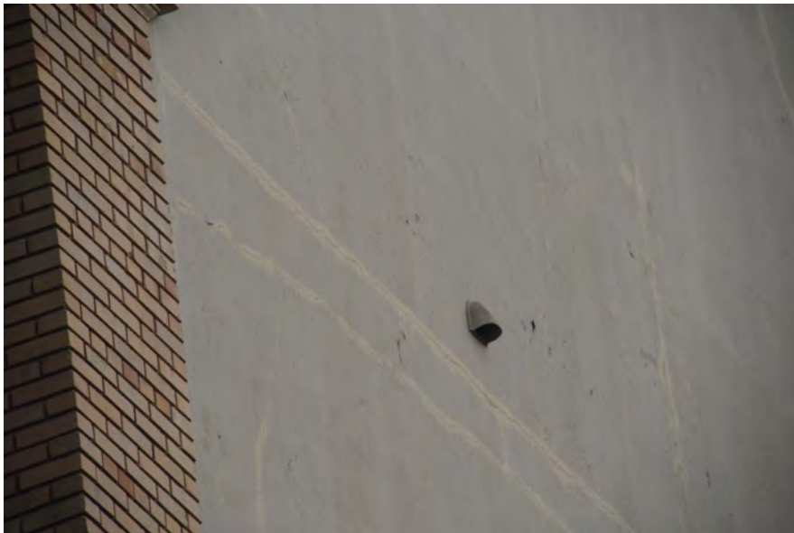
E - 24: Cracks at floor lines
