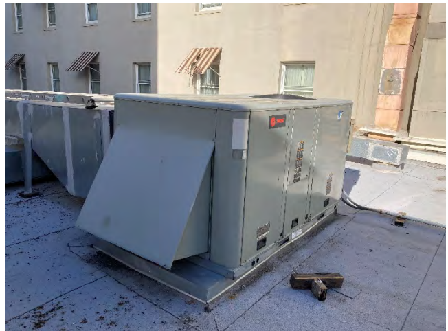
M-4. 20-ton packaged air conditioner.
