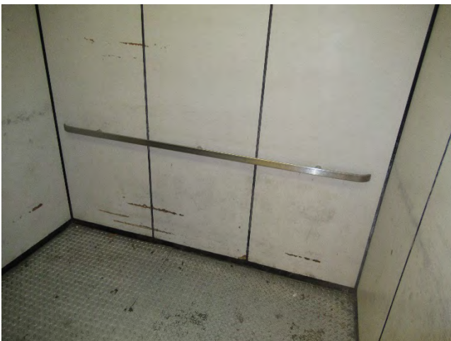
101. Floor and wall finishes in the Kitchen elevator. This elevator is in poor condition and should be modernized.
