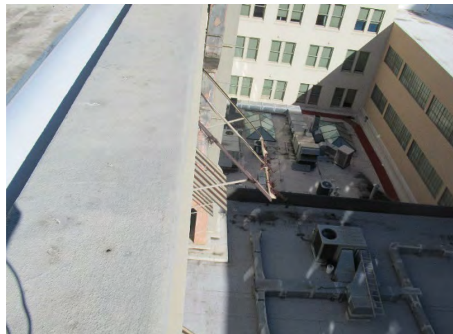
18. Several cloth awnings, installed over some of the courtyard windows are either missing or ripped. As an optional Modernization cost, the awnings and brackets should be replaced on windows where they were previously installed.
