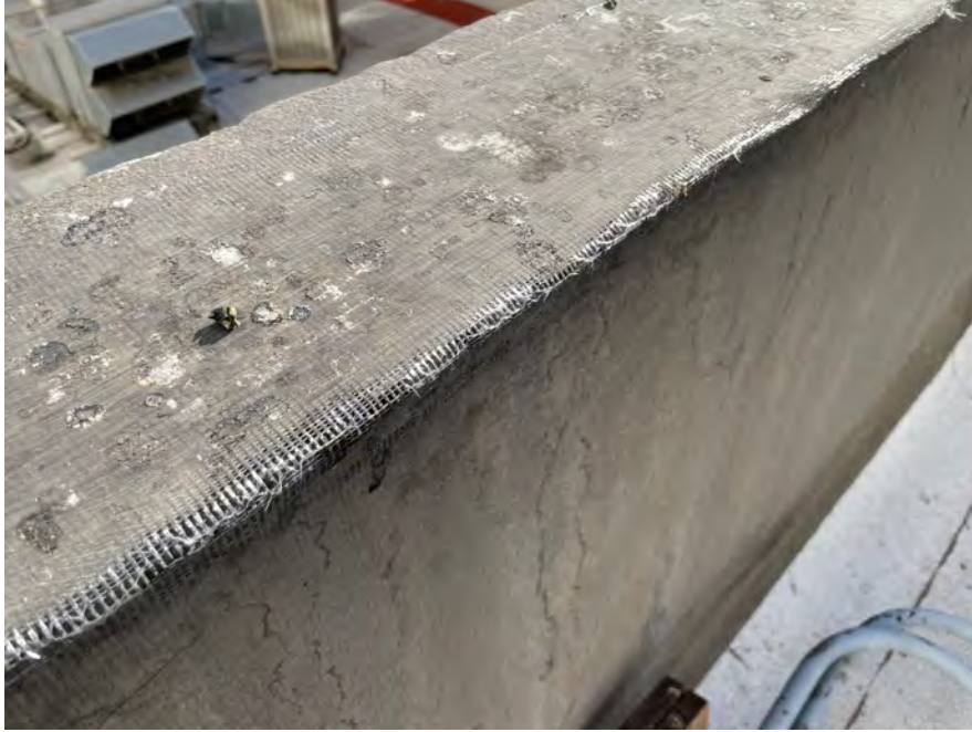
E - 21: Exposed reinforcement fabric
