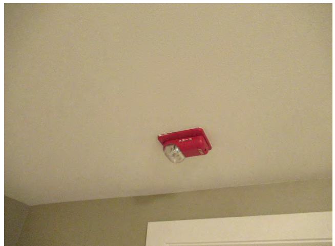
108. Fire alarm horn/strobes are provided in public restrooms.
