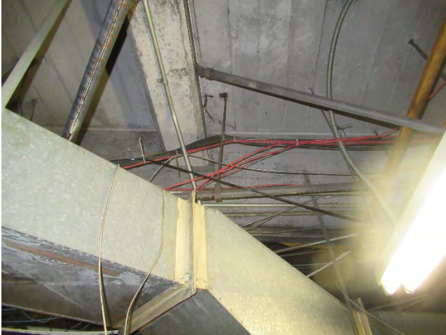
19. Building structure is framed with concrete girders and beams, with concrete floors.
