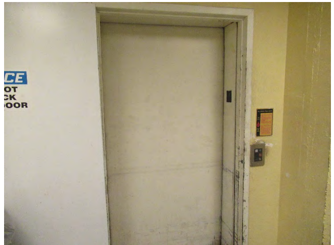
100. The Kitchen elevator in the basement.
