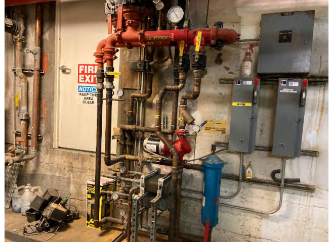
M-8. Hot water circulation pumping system.
