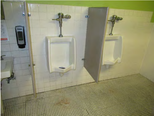
85. Men's locker bathroom. The urinals don't comply with Accessibility code.
