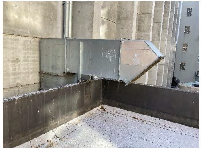
M-10. Underground parking garage exhaust termination.
