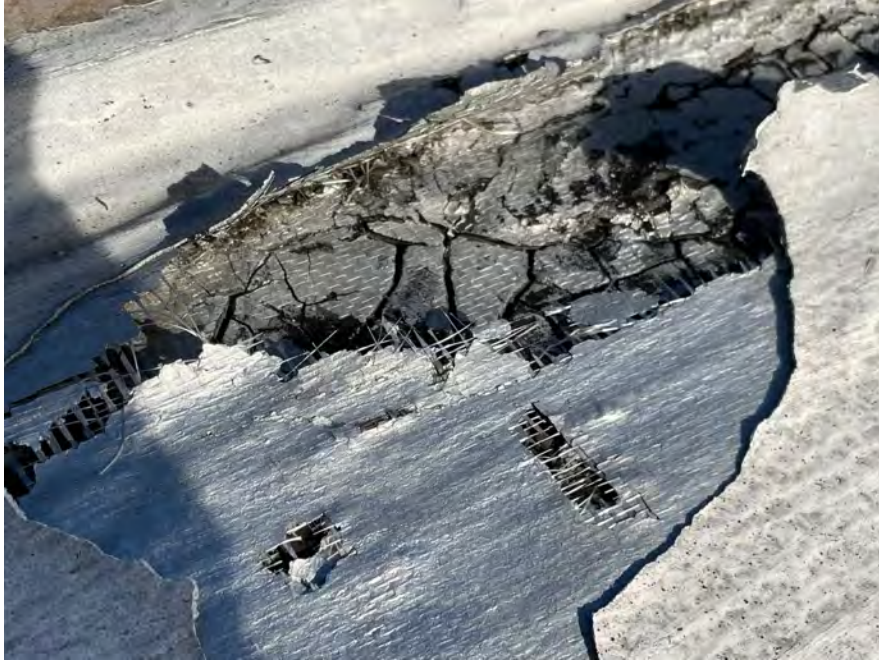
E - 5: Typical damage at Main Roof
