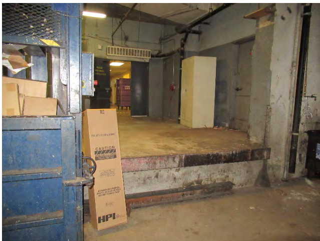
95. Trash compactor at the loading dock.
