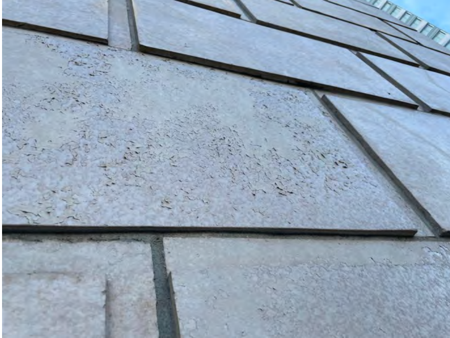
E - 27: Peeling paint on terra cotta
