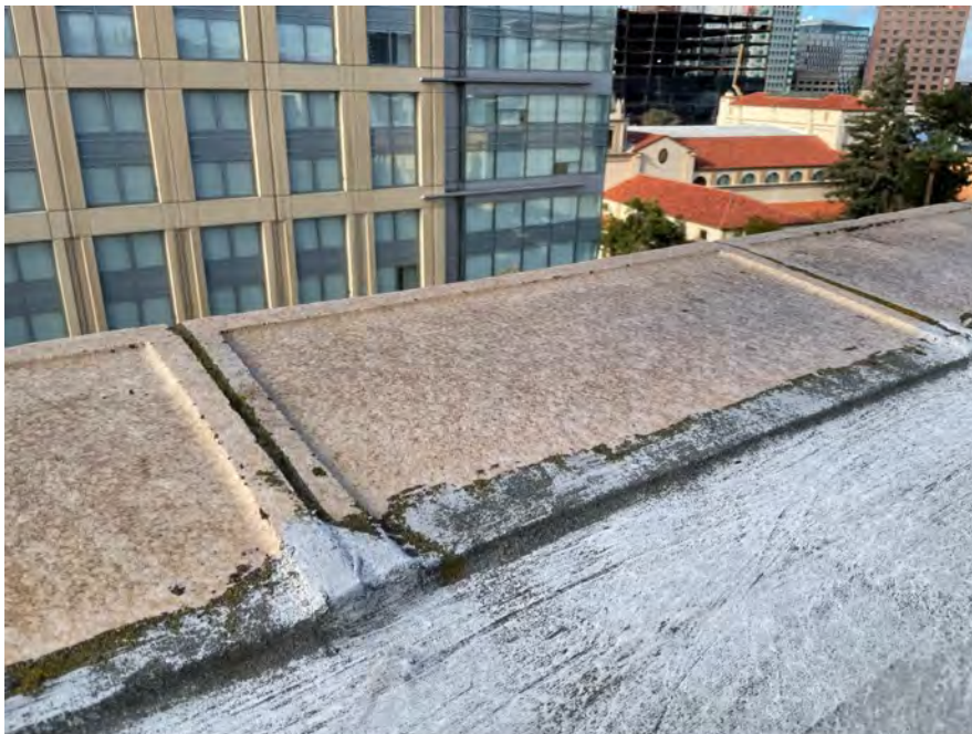
E - 6: Bio-growth at mortar and on coating
