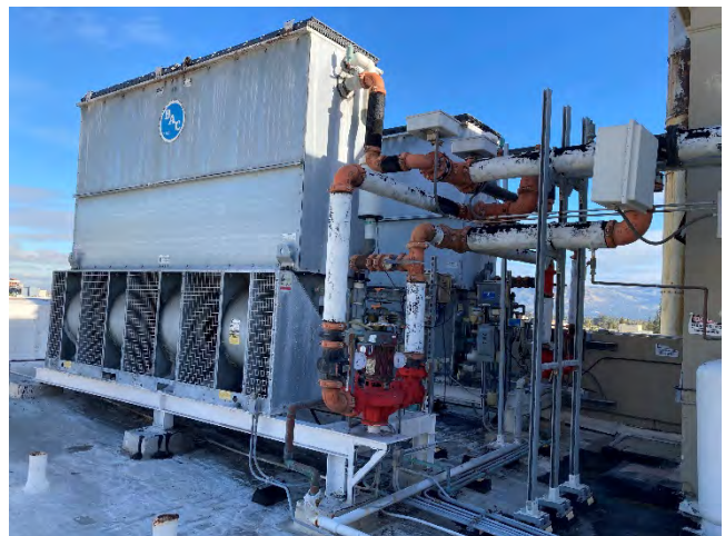
M-6. Condenser water loop evaporative condensers.
