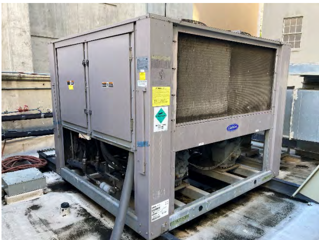
M-5. 45-ton air cooled chiller.
