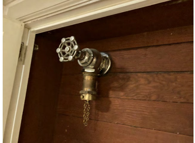
M-20. Corridor fire hose cabinet.
