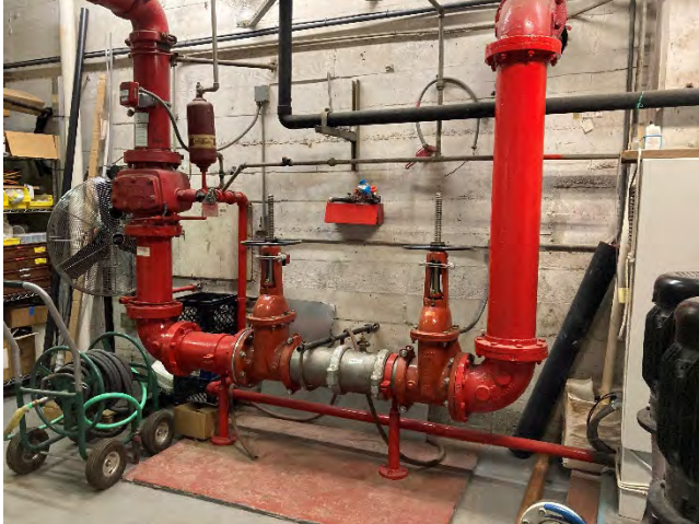
M-19. Fire sprinkler water service with backflow preventer.
